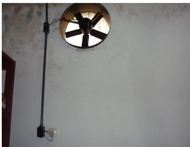
Exaustor do Almojarifado
